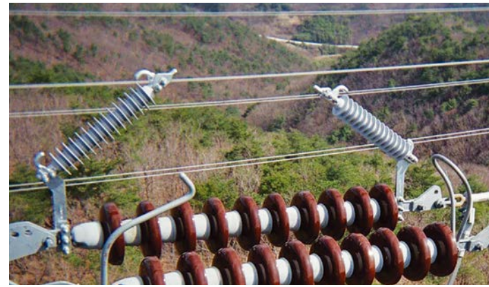
피뢰기설치장치 Attached to Arrester
